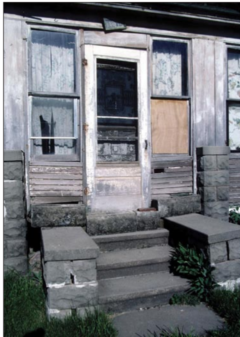
Rundown housing creates a nuisance in some communities.
